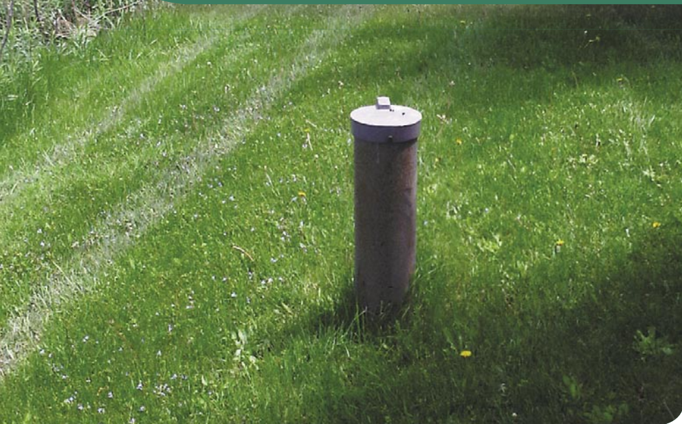
Small Drinking Water System at the Stoneridge Conference Centre Well.
